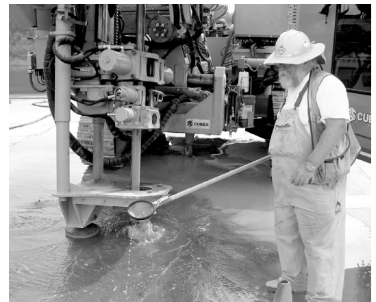
A geologist observes cuttings produced by a Cubex drill during foundation grouting upstream of the centerline of the earthen embankment of Wolf Creek Dam.
